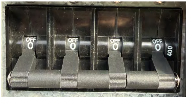
Figure 3.2 Battery overcurrent protection device (breaker)
