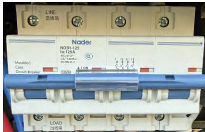
Figure 3.1 Backup port overcurrent protection device (breaker)
